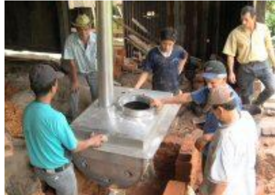
Installing appropriate technology on an organic farm Photo from the CADO archives
